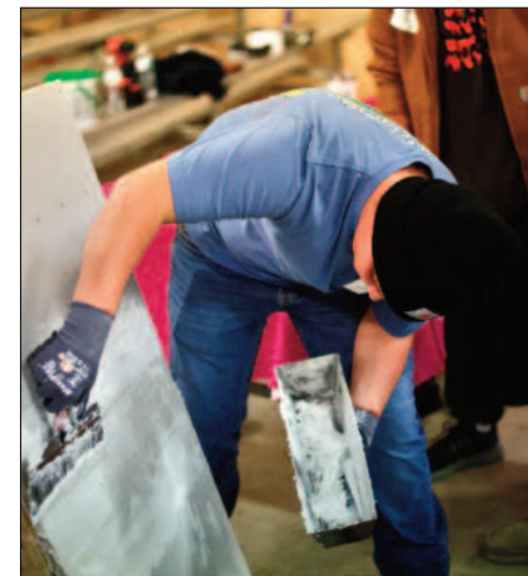
Adena Corporation taught teens how to apply drywall mud and each of them could practice doing it. Photo courtesy of Elliot Wall.
